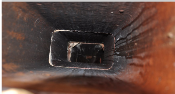
Rain entering the chimney
