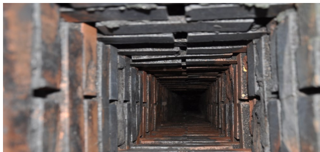
75% of mortar has been eroded away due to weather
