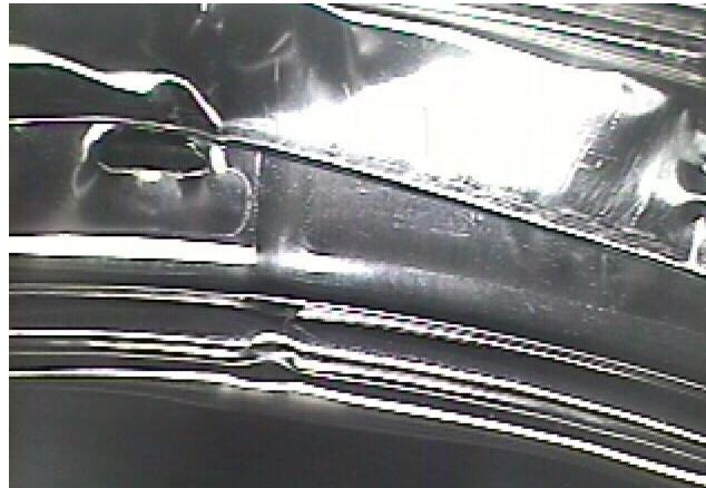
During construction the prefabricated chimney liner was not connected properly
