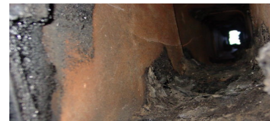
Pyrolyzed creosote and cracked flue liner
