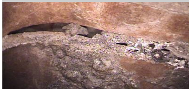
Open Mortar joint - Exhausting combustibles into wrong area outside the chimney
